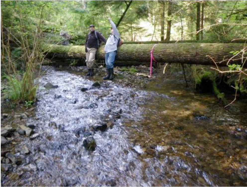
Site 5. – Large fir log is to be cut at approximately the ribbon point and allowed to fall into the stream. The root wad (hidden to the left) will anchor the log.
