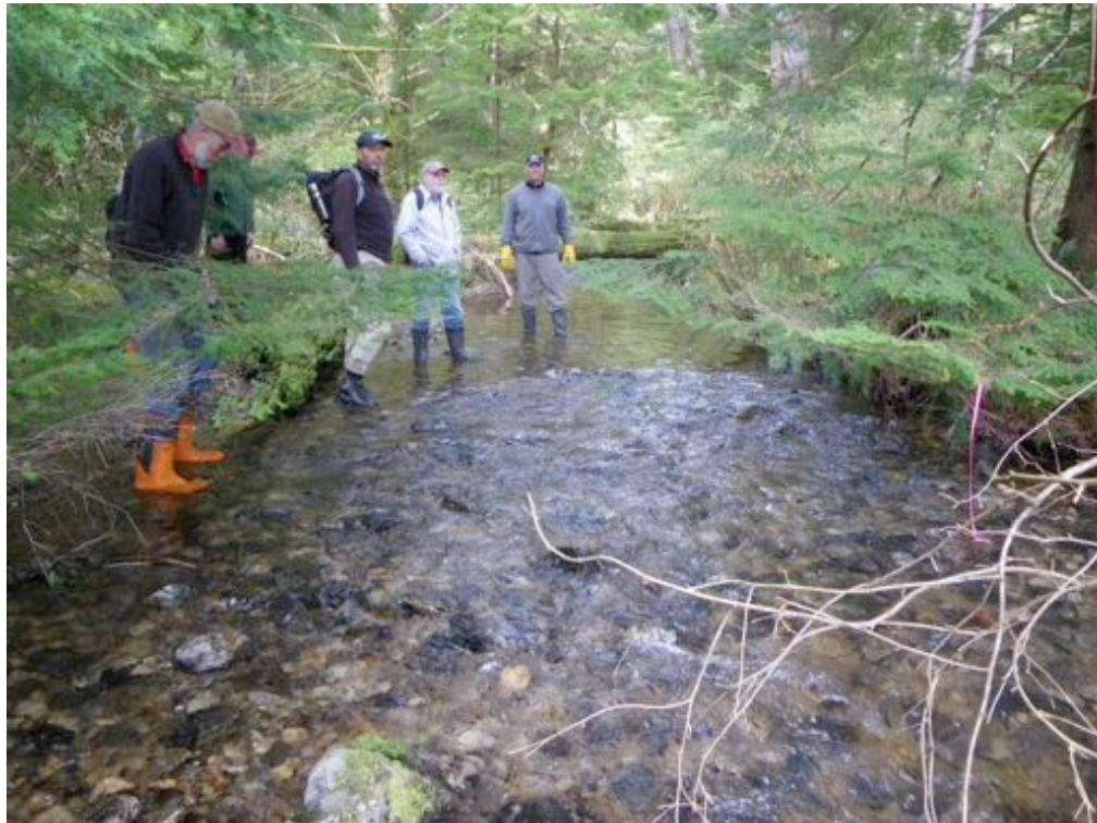
Site 2. – Site for a two log deflector installation. Each deflector extending \frac{2}{3} distance into stream bed, spaced 2 m apart.
